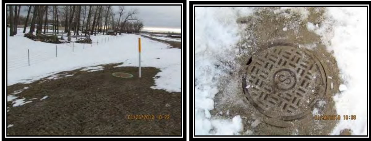
Figure 4: Toe Drain Pump Basin and Cleanout
