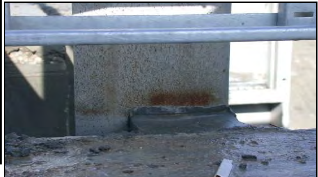
Contamination by nails left on the surface
