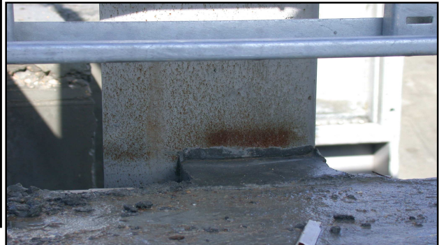
Contamination by nails left on the surface
