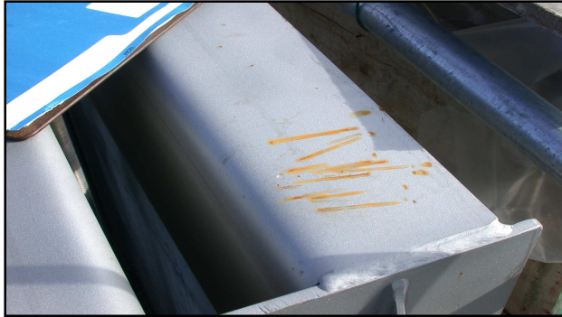
Contamination caused by grinding nearby
